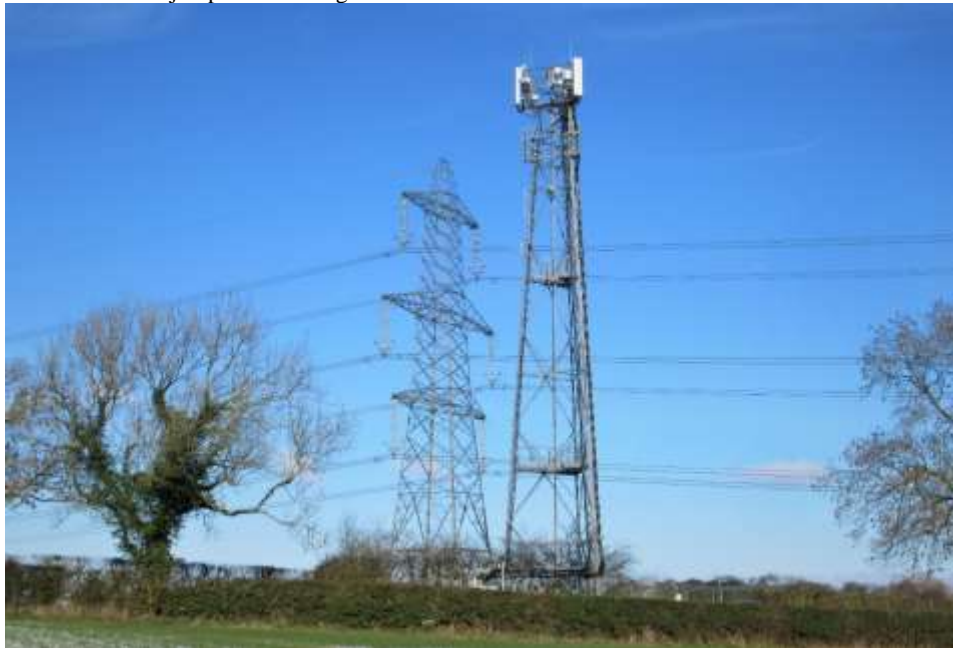
High voltage powerlines with a mast for microwave signals. A formidable combination. Easingwold, North Yorkshire, England. Photo by author.
