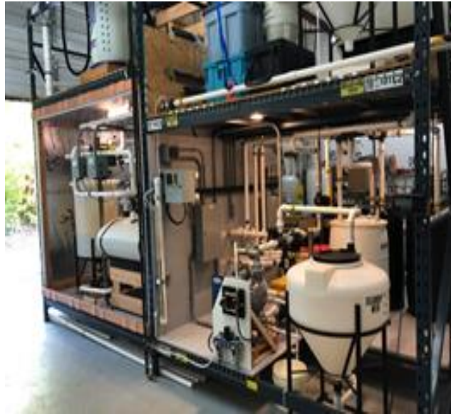
Figure 2. MEF Pilot Plant
